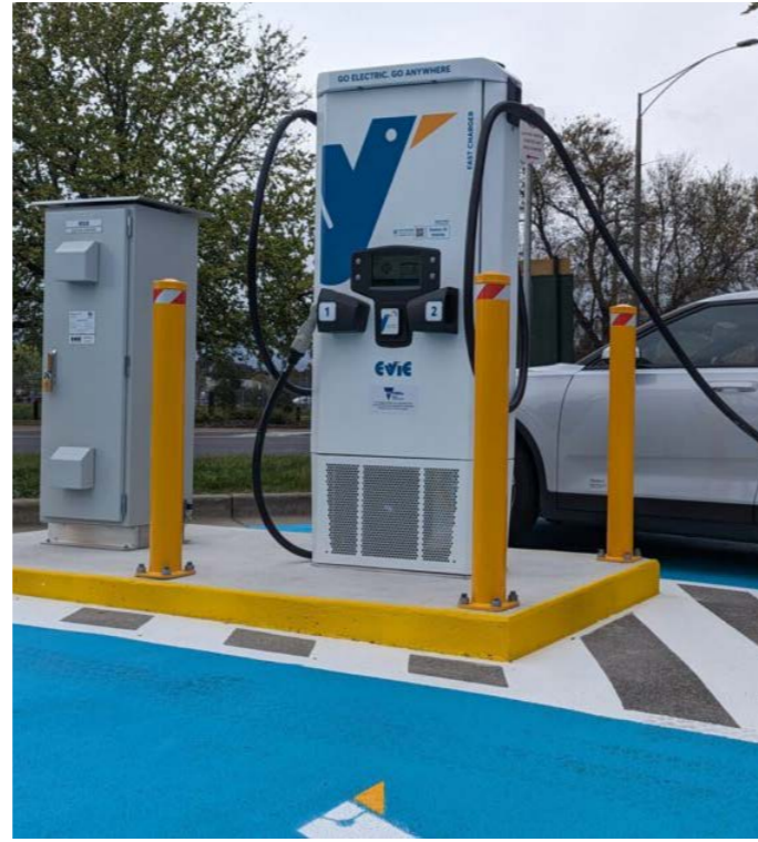
EV Charging Station
