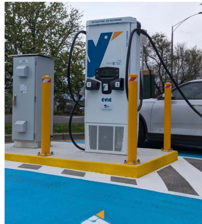
EV Charging Station
